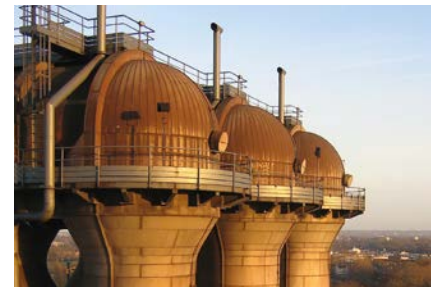
Blast furnace / stove dome
